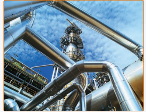
Chemical, Oil and Gas
