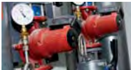
Actuators, valves, control cabinets
