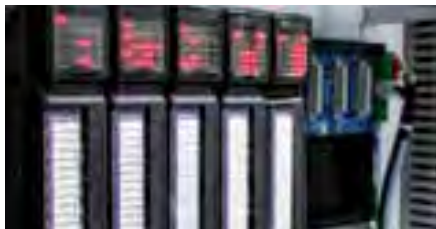
Connections to PLC
